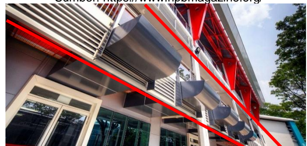
Gambar 7. Pipa Cahaya Horizontal Gedung BCA Academy, Singapore
