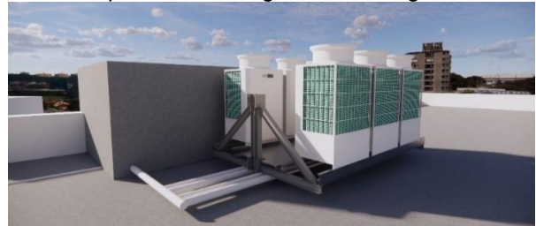
Figure 6. VRF Outdoor Units (Source: Author, 2023)
