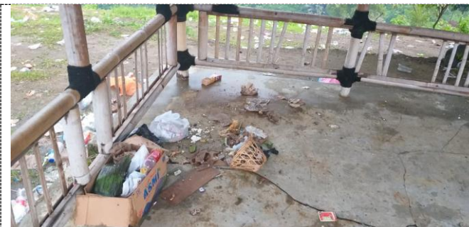
Figure 8. Gazebo's Condition In The Harvesting Area.
